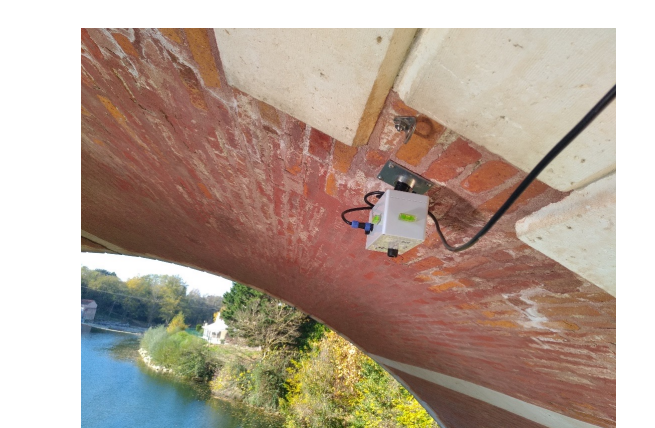
Figure 6 Illustration of a vortX.io μVTX-1 installed in the south of France
