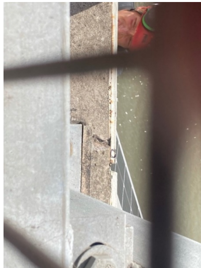
Figure 17: Reference point for vertical alignment - Black circle on white lip to concrete footing to pedestrian pathway barrier
