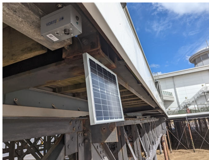
Figure 18: Micro-station and solar panel installed in Weston-Super-Mare
