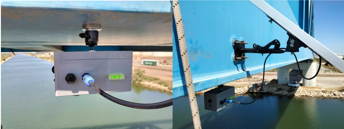
Figure 15: Micro-station and solar panel installed in Fos-sur-Mer
