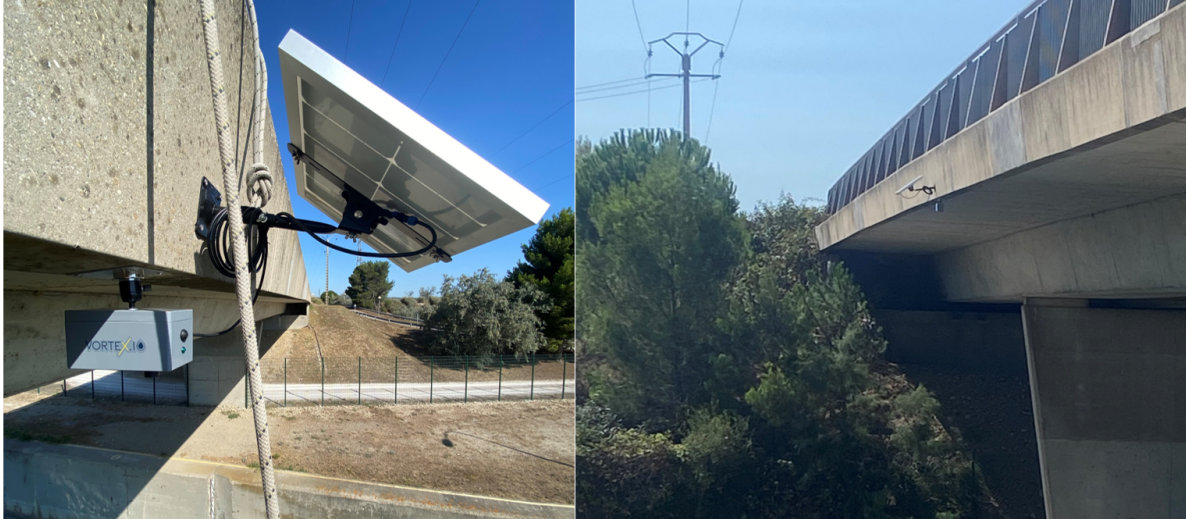
Figure 14: Micro-station and solar panel installed in Port-Saint-Louis-du-Rhône
