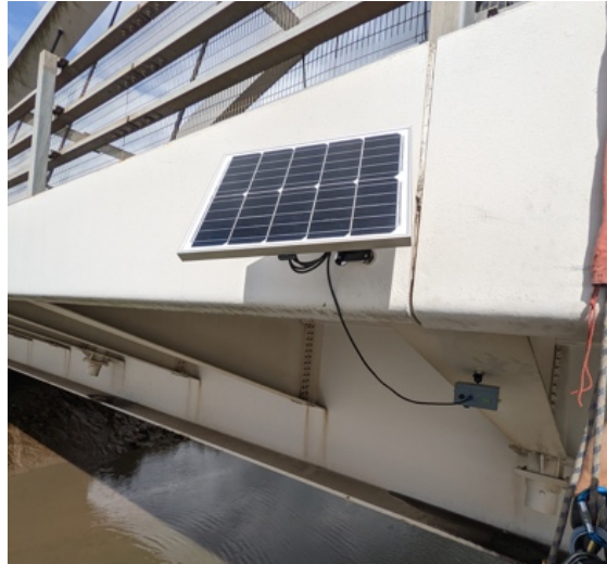
Figure 16: Micro-station and solar panel installed in Newport
