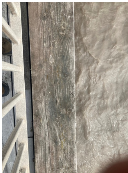
Figure 19: Reference point for vertical alignment – cross marked on wooden beam behind and below pedestrian barrier
